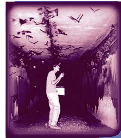
Bat Conservation International’s Brian Keeley observes Cave bats roosting inside a TxDOT highway drainage culvert in South Texas. Photo by Annika Nicklaus.
